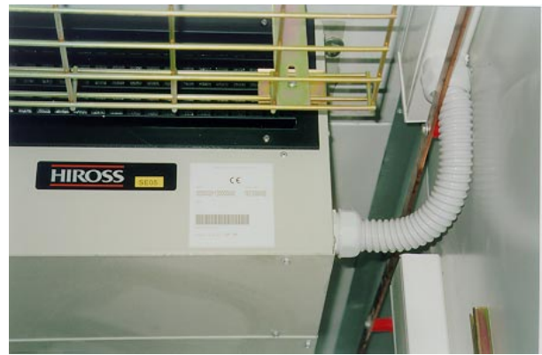
Fig. F – Details of the SE electrical connections with cable presser and plastic sheath (not supplied by us)
