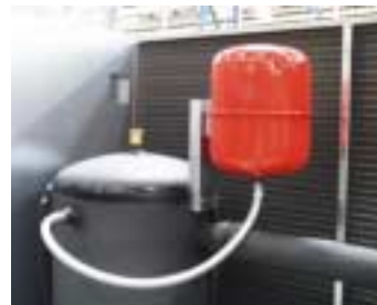
Chilled water Expansion vessel
