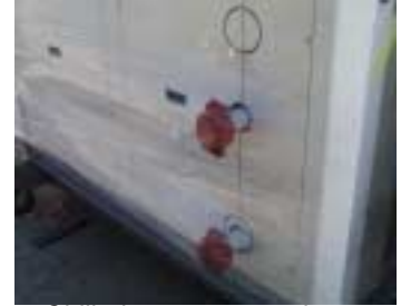
Chilled water connections
