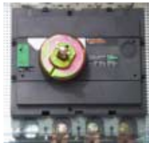
Main ON/OFF switch
