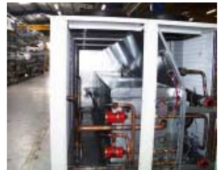
Compressor acoustic enclosure
