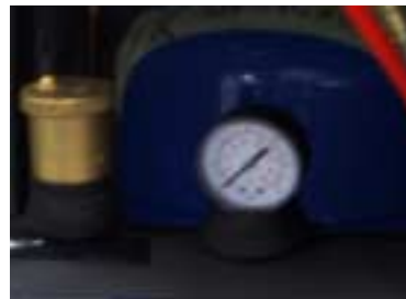
Water Pressure Gauges
