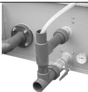
Drain pan system in air washer chamber
